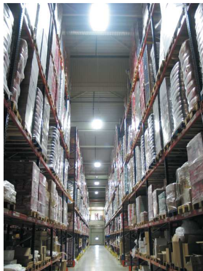
BLADE 380 R60 Deluxe COR HBPIR with energy consumption from 76 to 255 W each after. Height 10-12 meters.
