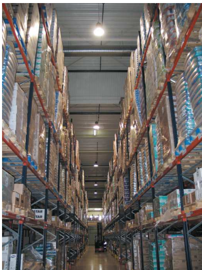
Highbay fittings with metal halide tube and energy consumption of 440W each before. Height 10-12 meters.
